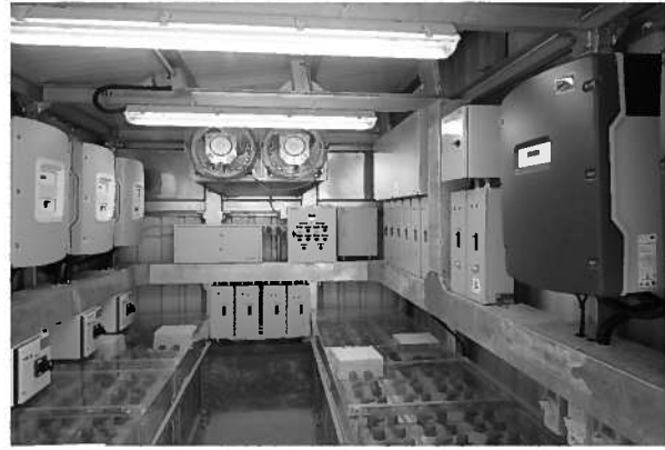
Fig. 3. Interior of Phase 1 Plant Room
